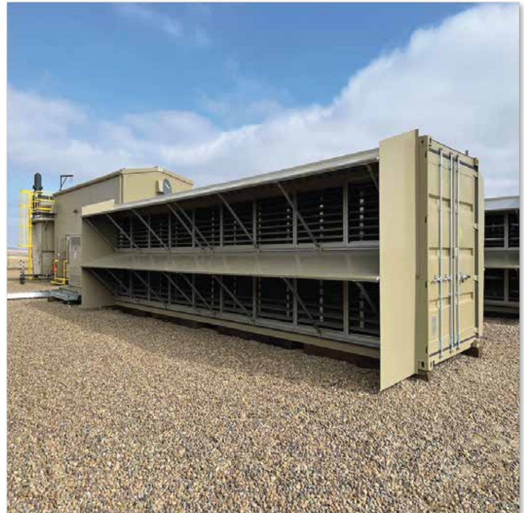
Digital flare mitigation system
